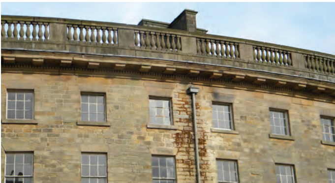
A sorry site - the rear of Buxton's Crescent which is vastly superior architecturally to the rear of the Royal Crescent at Bath.
